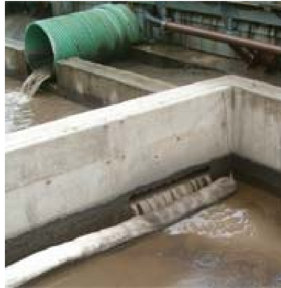
“Clean” water overflow wier and oil skimmer
