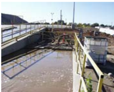
Water drains into a settlement pit where it is collected for treatment and re-circulation to the wheel wash
